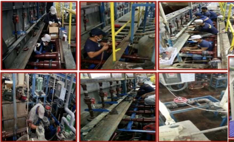
Maintenance Production line
